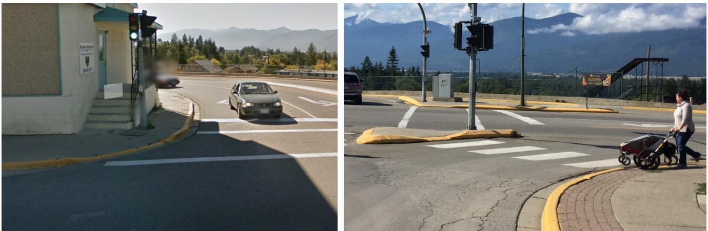
Narrow sidewalk at southeast corner of Canyon Street and Cook Street (left) and poorly designed cut through median / island at the northwest corner (right).
